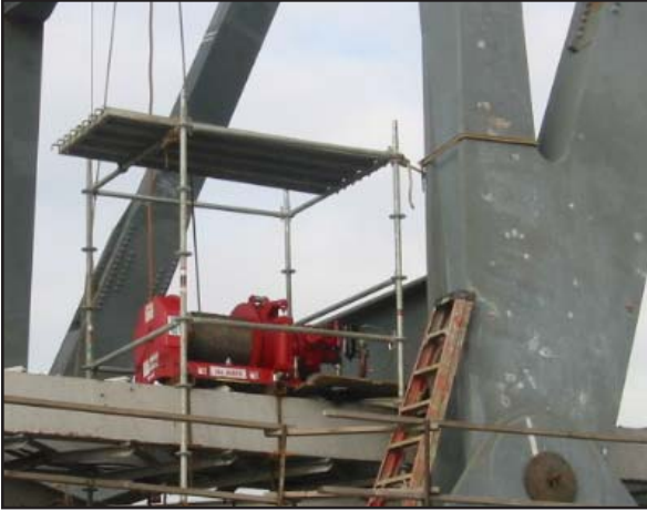
Above: TA winches like the one shown above were positioned on the base piers, raising and lowering iron crossbeams during the refit.
