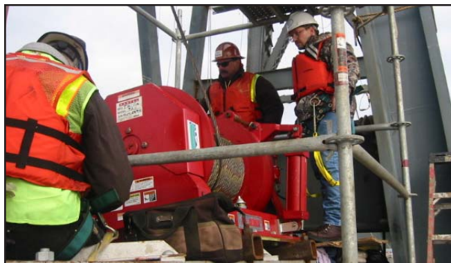
L to R: Gene Rosamilia of Koch Engineering, and Bill Sievers and Jim Abts of Thern inspect the setup of a TA series winch.
