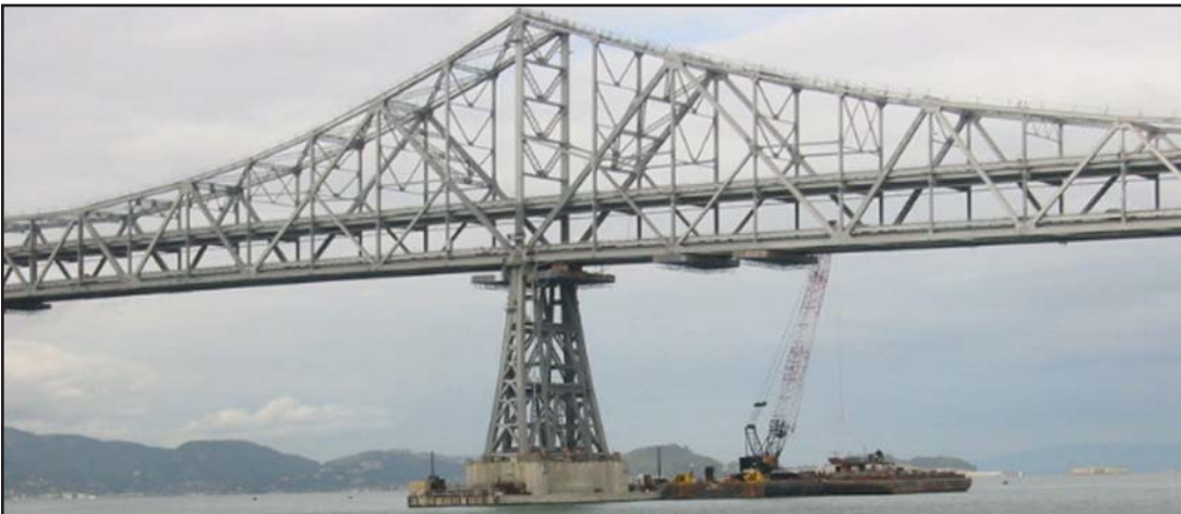
A utility barge works on the superstructure of one of the base piers of the bridge.
