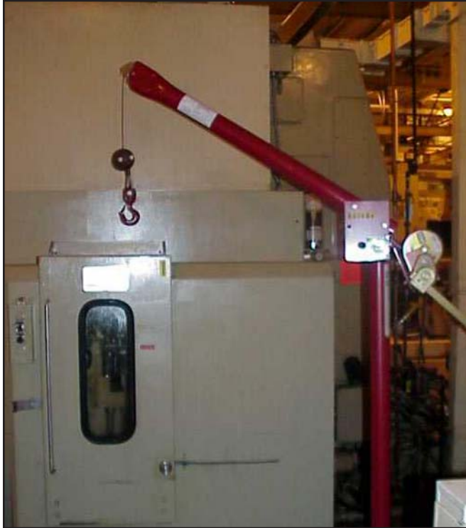
A Thern 5122 davit crane at the Pratt & Whitney facility.
